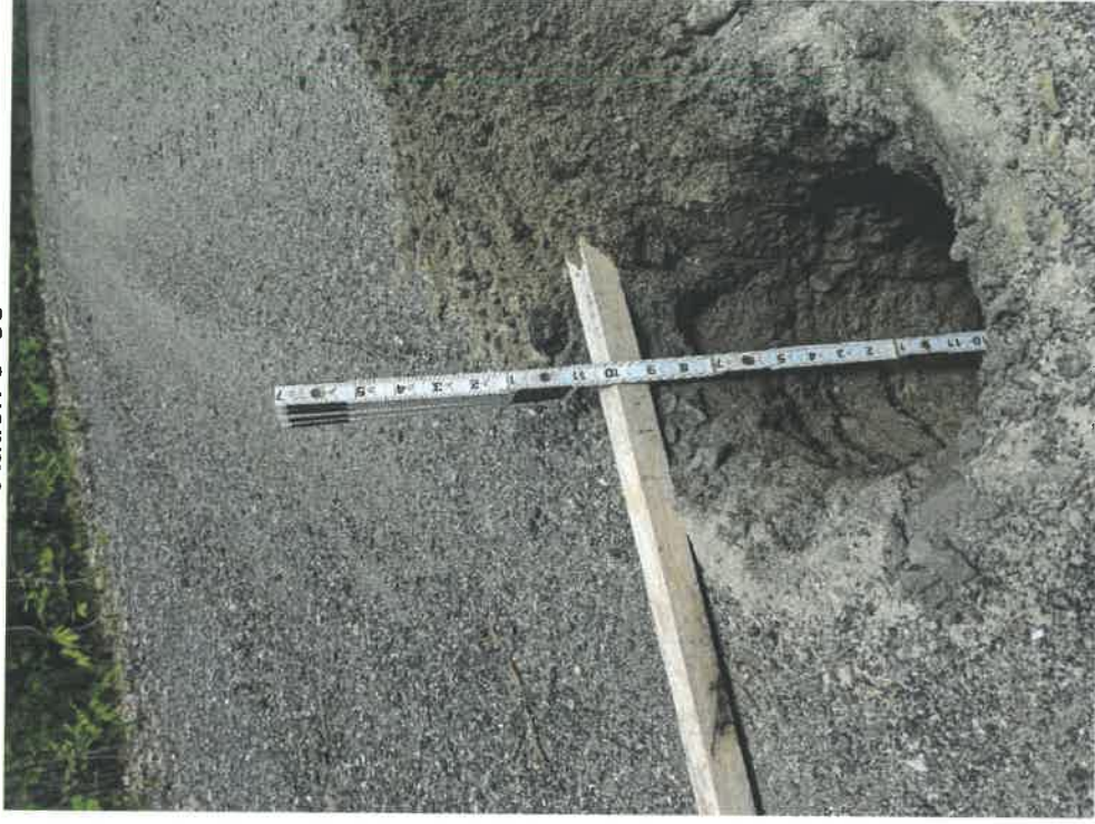
Gravel Depth: 21" Road Width: 22'±
