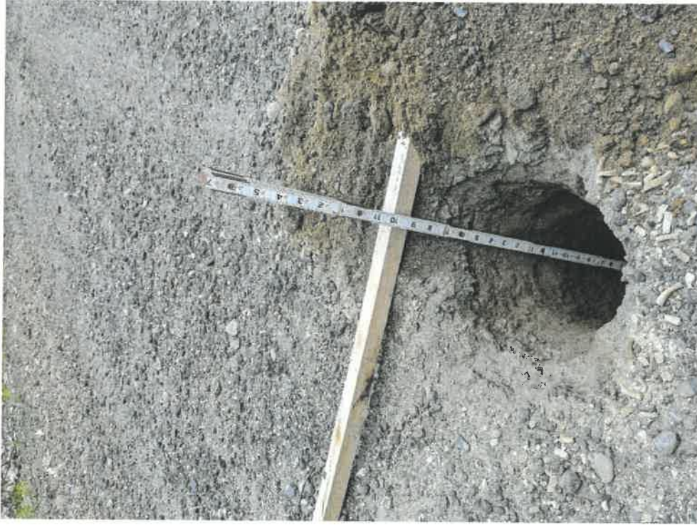
Gravel Depth: 21" Road Width: 23'±
